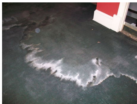
Damage to lounge floor due to a pipe cracking on the water heater.
